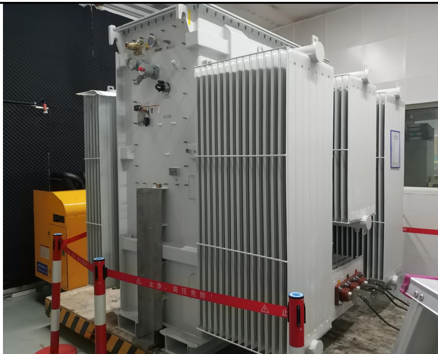
Figure 3 Image of the transformer under test
